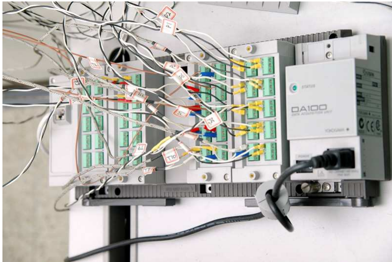
Fig 2.9 Photograph of data acquisition system
