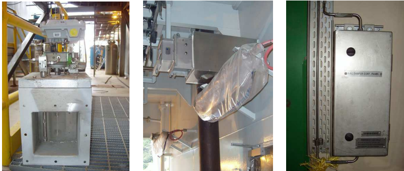
Fig. 4.6 Fire damper and local control panel
