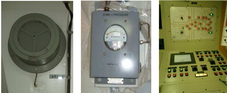
Fig. 4.24 Pressure control valve and monitoring system for naval ship
