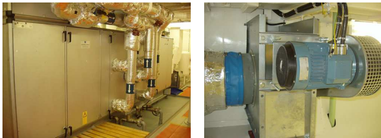
Fig. 4.14 Air Handling Unit and re-circulation fan
