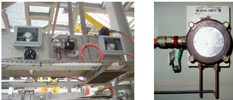
Fig. 4.7 Combustible gas detector and Pressure differential device
