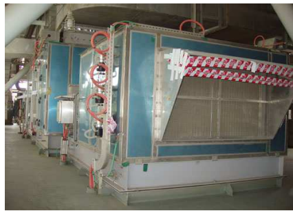
Fig. 4.4 Pressurizing unit and air handling unit for living quarters
