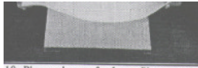
10. Place a layer of release film over the laminate. This layer should overhang the laminate on each side by at least 3 to 4 inches (8 to 10 cm). The release film layer allows volatiles to escape while containing resin.
