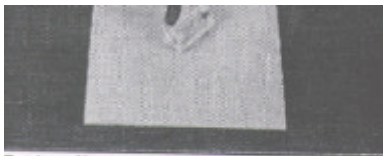
7. A roller may be used to remove any trapped air bubbles and wrinkles from the layup.
