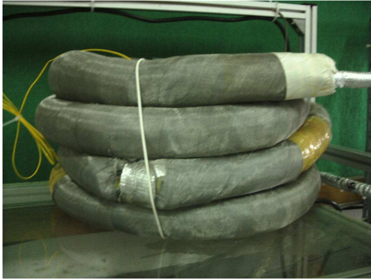
Fig. 3.5 Photograph of Pre-heater
