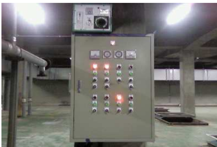
Fig. 3.3 Y-TURN process control panel used in this study
