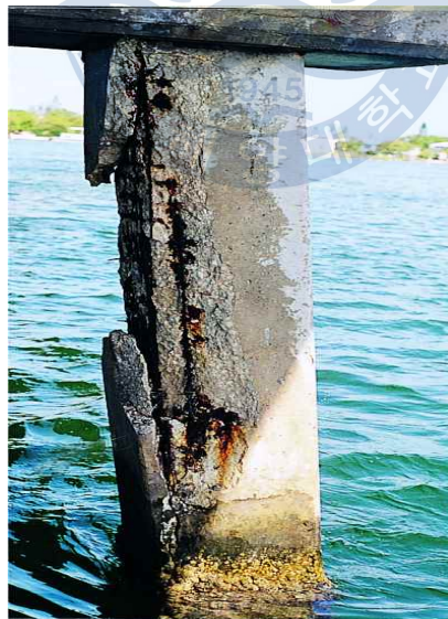
Fig. 1.1 View of the damaged splash & tidal zones in the marine bridge column [3]
