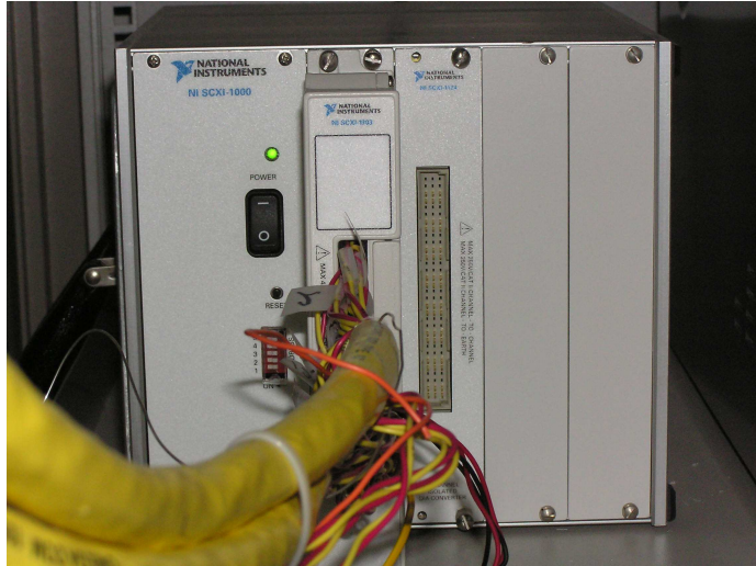
Figure 3. 11 Data acquisition system (NI Co.)
