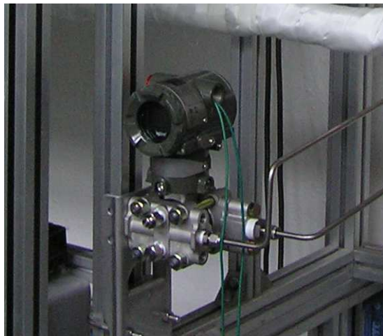
Fig. 3.6 Photograph of pressure drop transmitter
