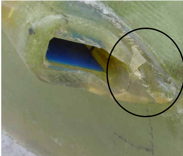
(a) Crack occurred under uncured condition
