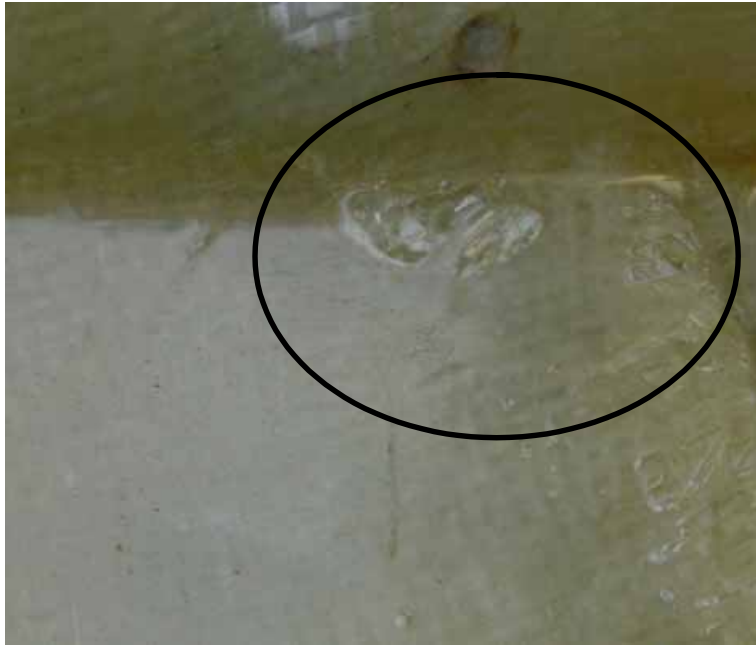
(c) Surface defect by bubble
