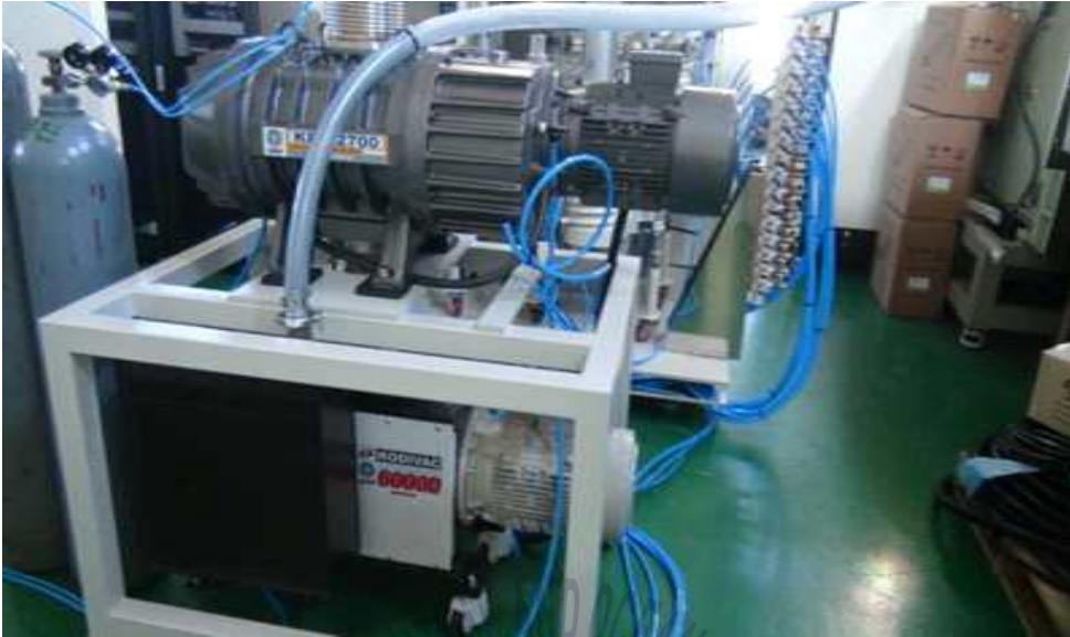
〈Fig. 3.4〉 The actual connection state of the rotary pump and booster pump
