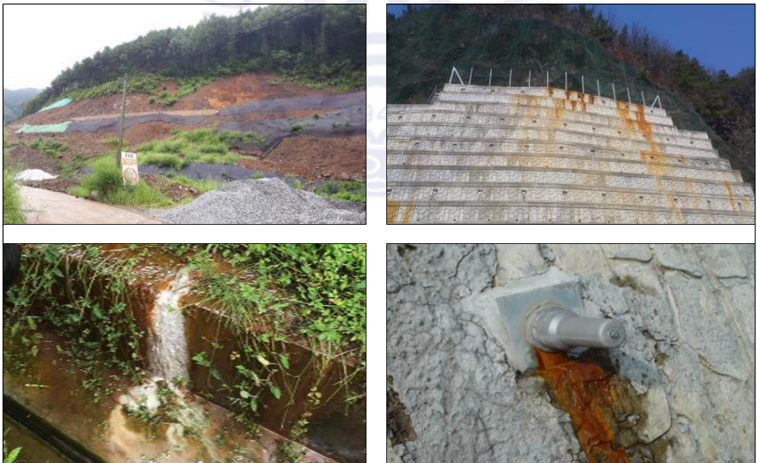
Fig. 1.1 Damaged cut slope and structure by acid rock drainage
