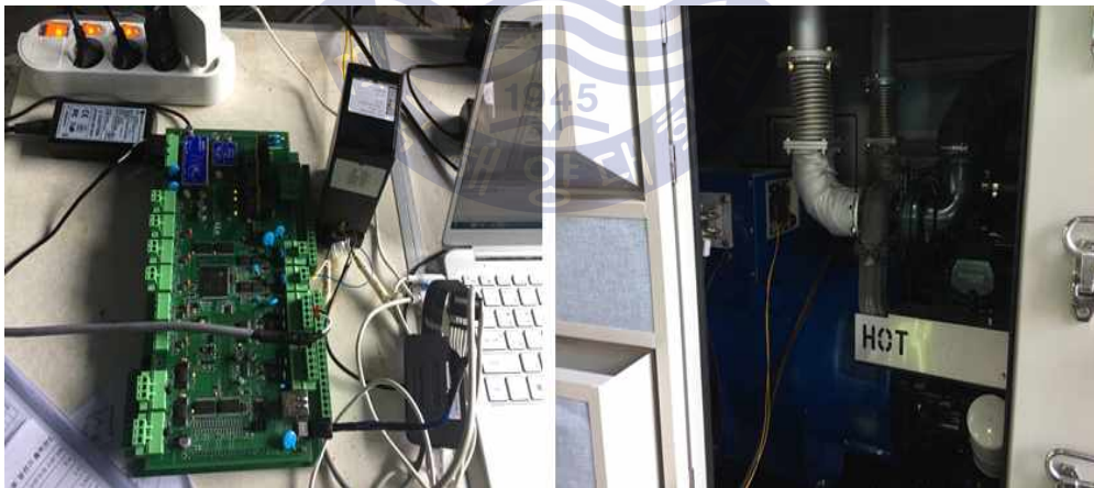
Fig 5.6 PMS & Potentiometer(Left), AVR of Diesel generator(Right)
