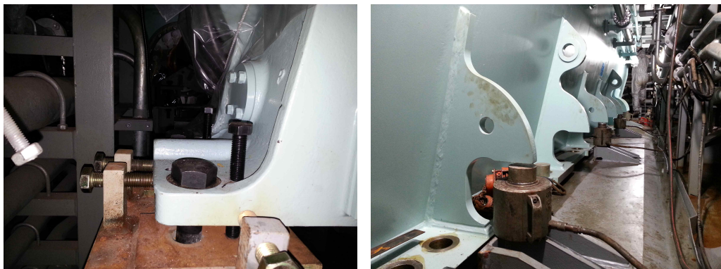
Fig. 3.5 Example of bearing offset adjusting device for intermediate shaft bearing (left) and Main engine (right)
