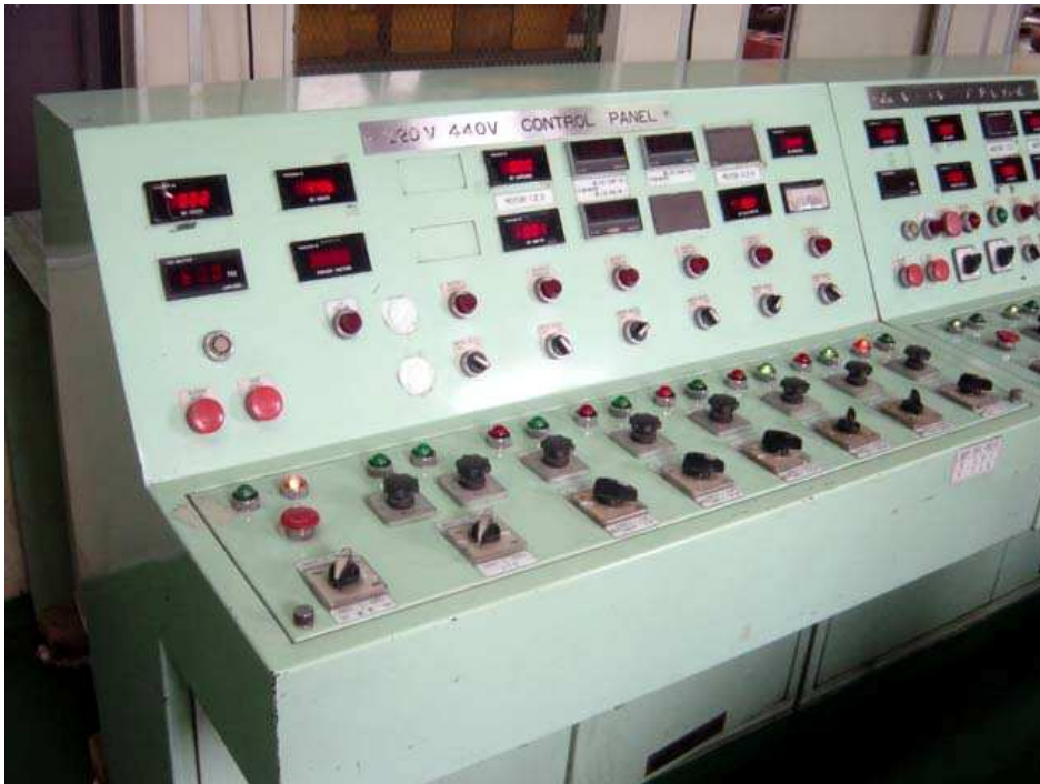
Fig. 3.7 Control panel(Watt Meter)
