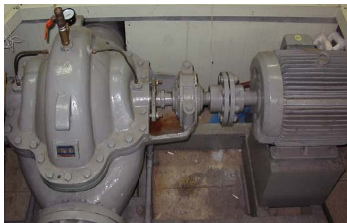
Fig. 3.3 Current generating device - Pump
